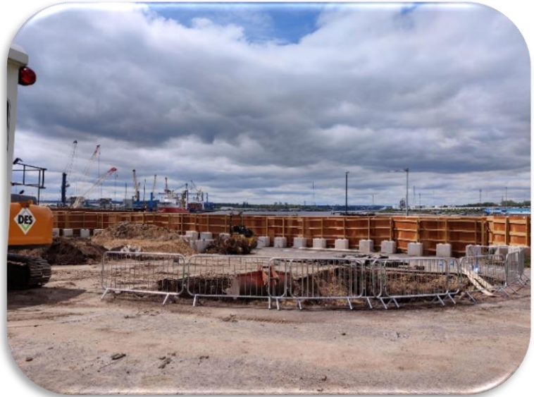
Holborn Renewable Energy Enabling Works Site
